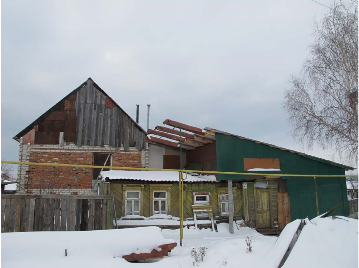
Photo 17. Although by local standards otkhodniks receive good wages and can afford to improve their living conditions, most of them cannot build a big new house in one go. Typically, having accumulated a certain amount of money the otkhodnik repairs part of the house or extends it. Then the money runs out. As soon as he saves a new amount, he extends the house further or repairs another part of it. This can go on for many years. The otkhodniks often pay little attention to the stylistic unity of the house and every time use different construction materials varying in color—those that are either cheaper or easier to purchase, or those that are at that time in trend. The photo shows a house with endless additions in Ardatov, Republic of Mordovia. Such buildings served as a certain beacon for us signaling the presence of an otkhodnik and helping us to find our respondents. Photo by Natalia Zhidkevich, November 2011.
